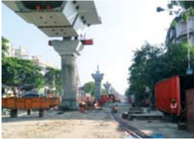
Work of extension of Metro Railway, Kolkata by Rail Vikas Nigam Limited.
