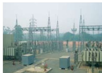
Chattarpur sub station of Delhi Metro Rail Corporation - IRCON project.
