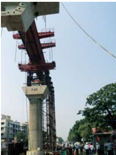
Work of extension of Metro Railway, Kolkata by Rail Vikas Nigam Limited.
