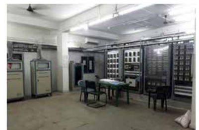
Relay Room of Gamharia station, SER
