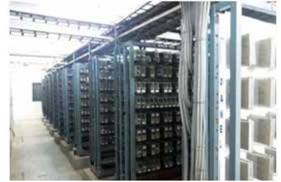
Relay Room of Gamharia station, SER
