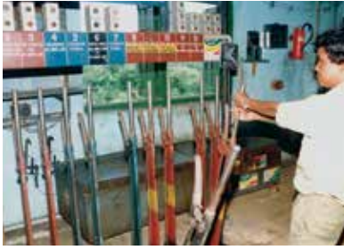
Route Relay Interlocking cabin
